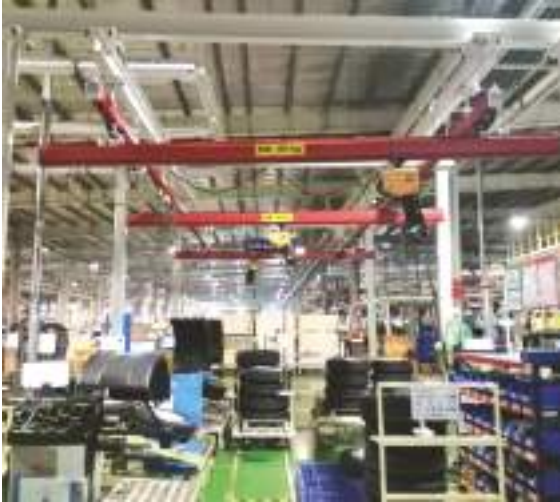
XY RAILS (STEEL) WITH HOISTS & STRUCTURE
