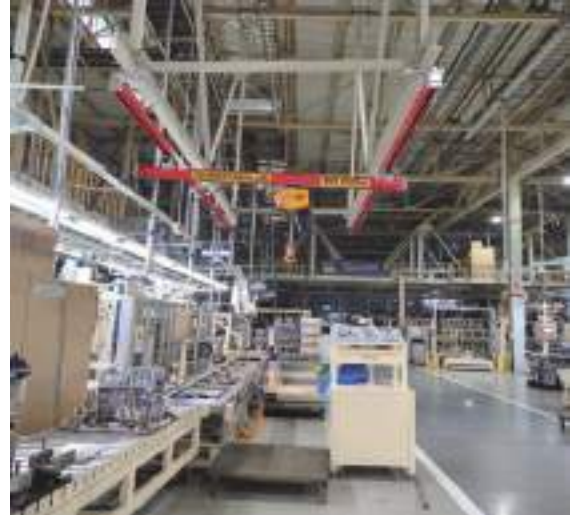
XY RAILS (STEEL) WITH HOISTS & STRUCTURE
