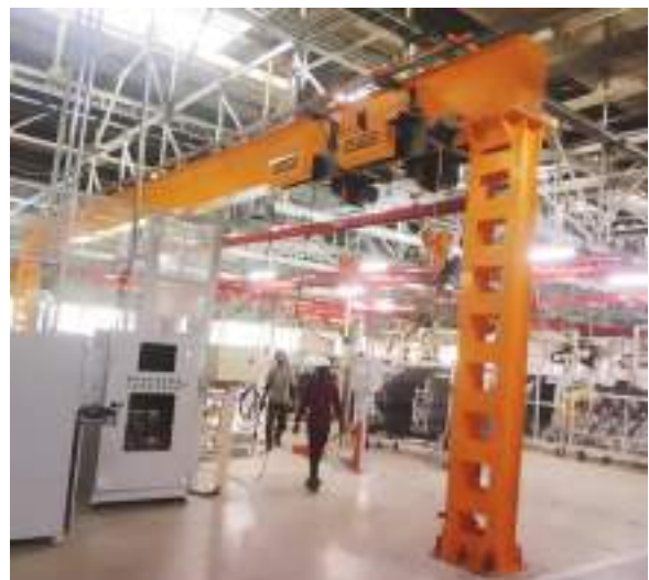
MONORAIL GANTRY CRANE-TANDEM OPERATION
